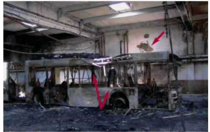
Fig.26.: The above arrow shows where the wall was leaked through by the exploded tank [24]
