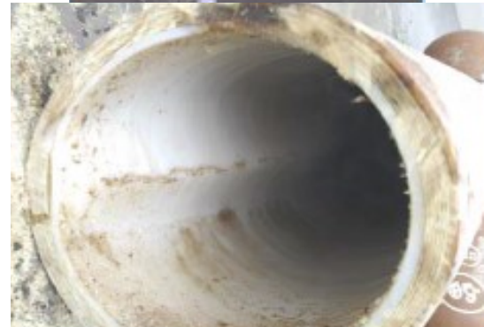
Fig.22.: The blistered liner can see on the above cut up cylinder, at low pressure the strung-out liner come off the epoxy-fibre layer, and the hydrogen accumulating between. On the lower picture the one already cracked liner is visible. The increase of the hydrogen passage through the wrapping resulted. [Source of the photo is uncertain]
